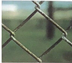
Galvanized Steel— 40% Rust, 60% White Corrosion
