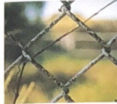
Galvanized Steel—60% Rust, 40% White Corrosion
