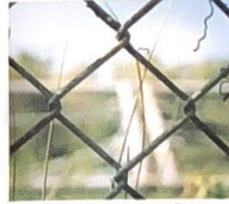
Aluminized Steel—10% Rust, 15% White Corrosion, 75% Gray
