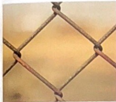
Galvanized Steel—100% Rust
