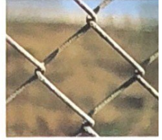
Galvanized Steel—5% Pinpoint Rust, 95% White Corrosion
