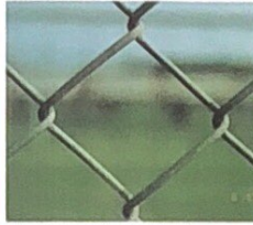
Aluminized Steel—2% Rust, 10% Metallic, 78% Gray, 10% White Corrosion
